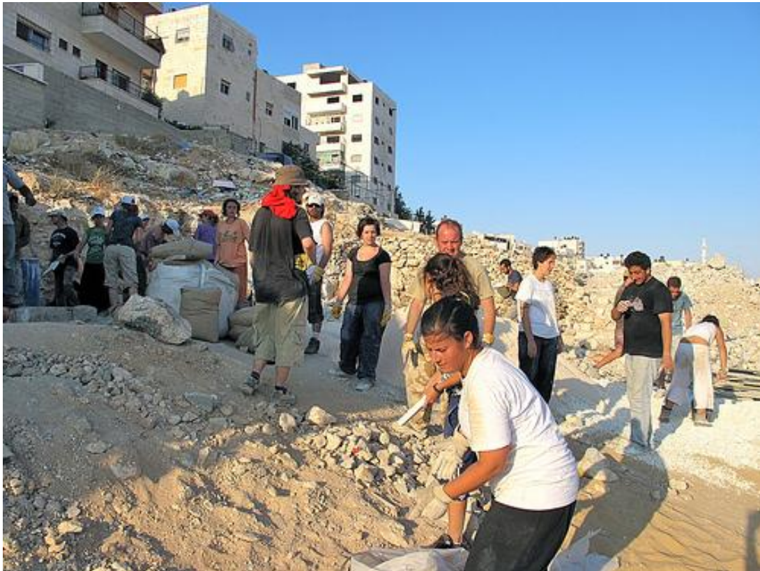
Volunteers from the Israeli Committee Against House Demolitions help to re-build the demolished home of a Palestinian family in East Jerusalem, West Bank
